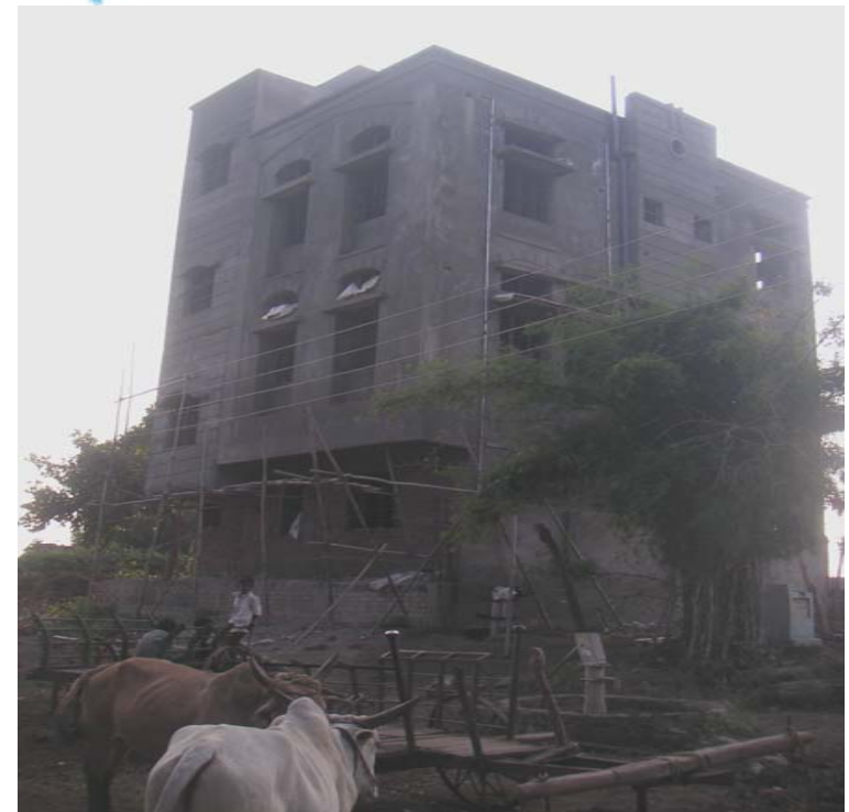
The Sangam's new purpose built Sub-Centre building in Narayanpur village nearing completion
